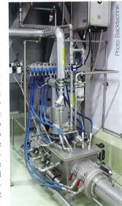
Flour, water, yeast and oil are mixed in the dough preparation unit and then are pumped into the maturation container.
