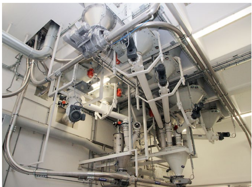
Discharge system with pneumatic conveying system
