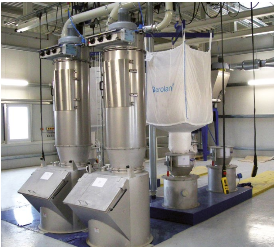
The feeding station for bags and big-bags is at the highest level of the mixing tower
