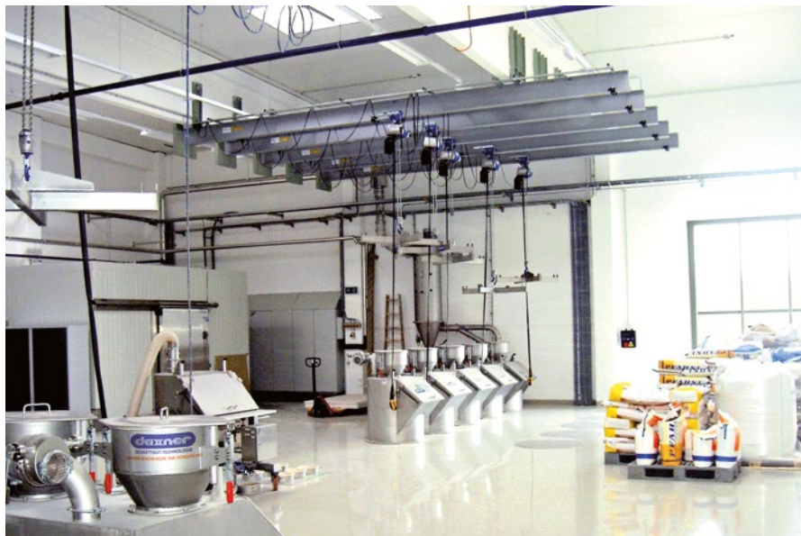
Intake station for ingredients in bags and big bags
