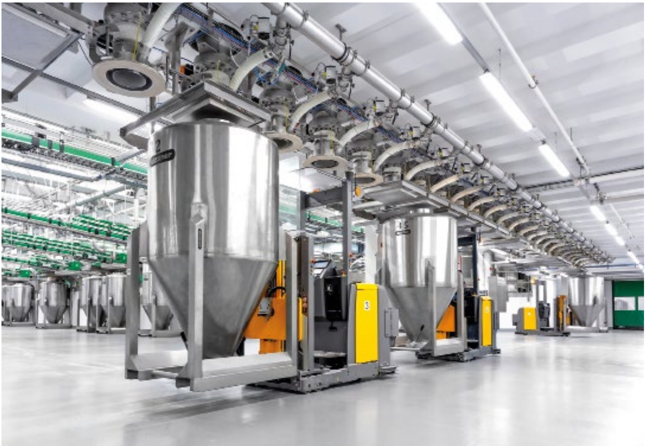
Fully automated collection system with Daxner Container Systems DCS in connection with the Automated Guided Vehicle system AGV Container series DCHD in hygienic design, volume capacity 1,200 ltr, CIP compatible
