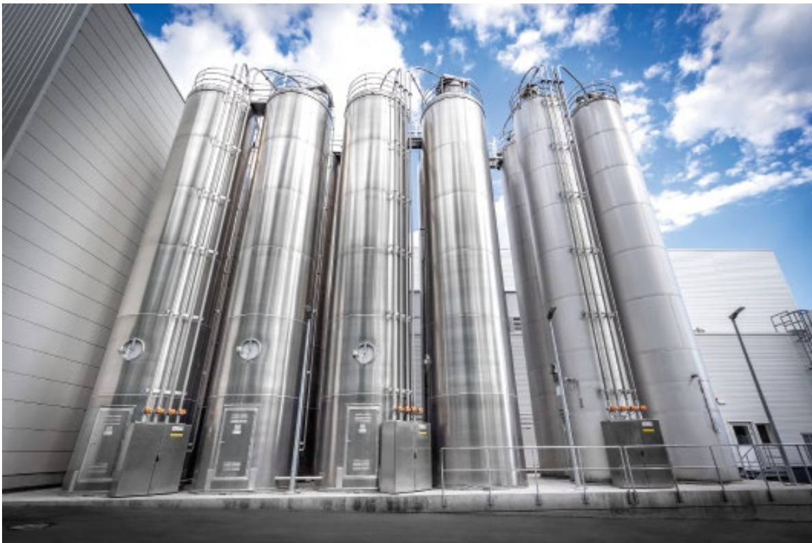
The main components are stored in outdoor silos and are conveyed pneumatically to the mixing lines.
