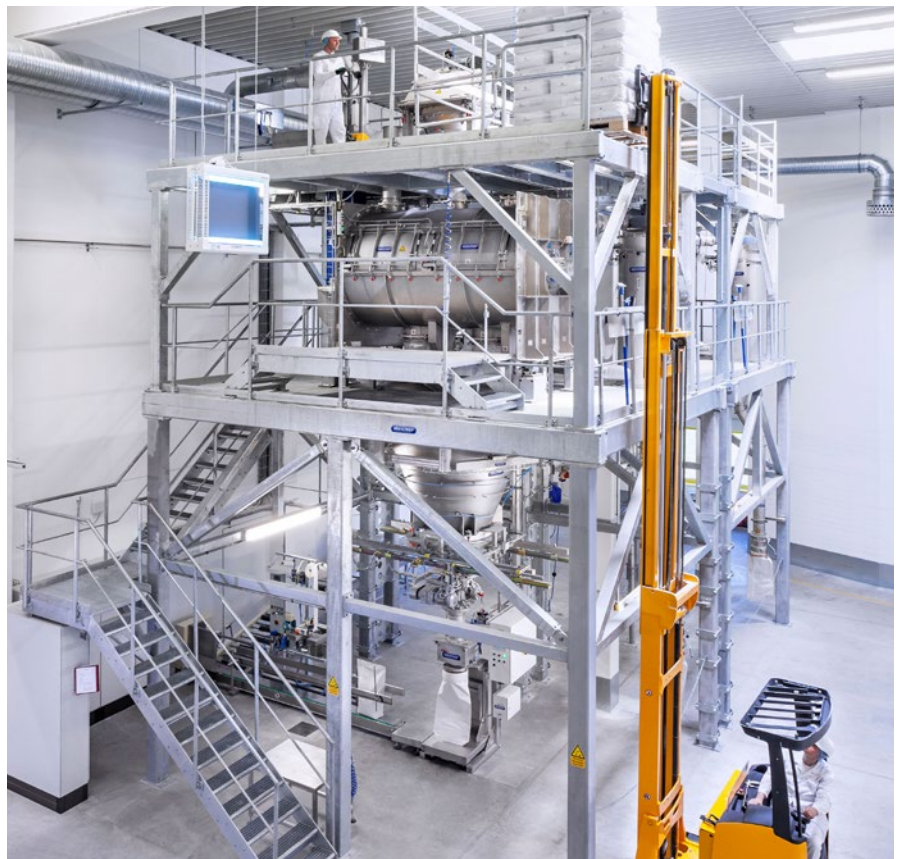
Both complete bags and pre-commissioned small and medium components are positioned onto the operating platform by a forklift truck
