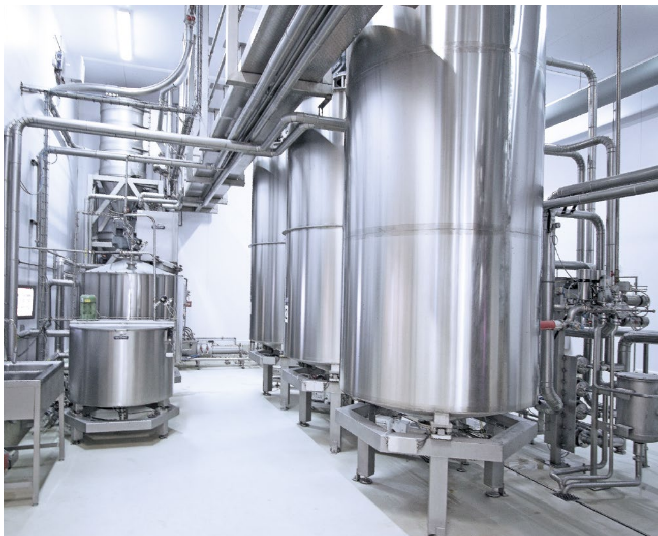
The plant made by Daxner International does not only convince visually, just as much expert knowledge is included in the technology and the intelligent control system.
