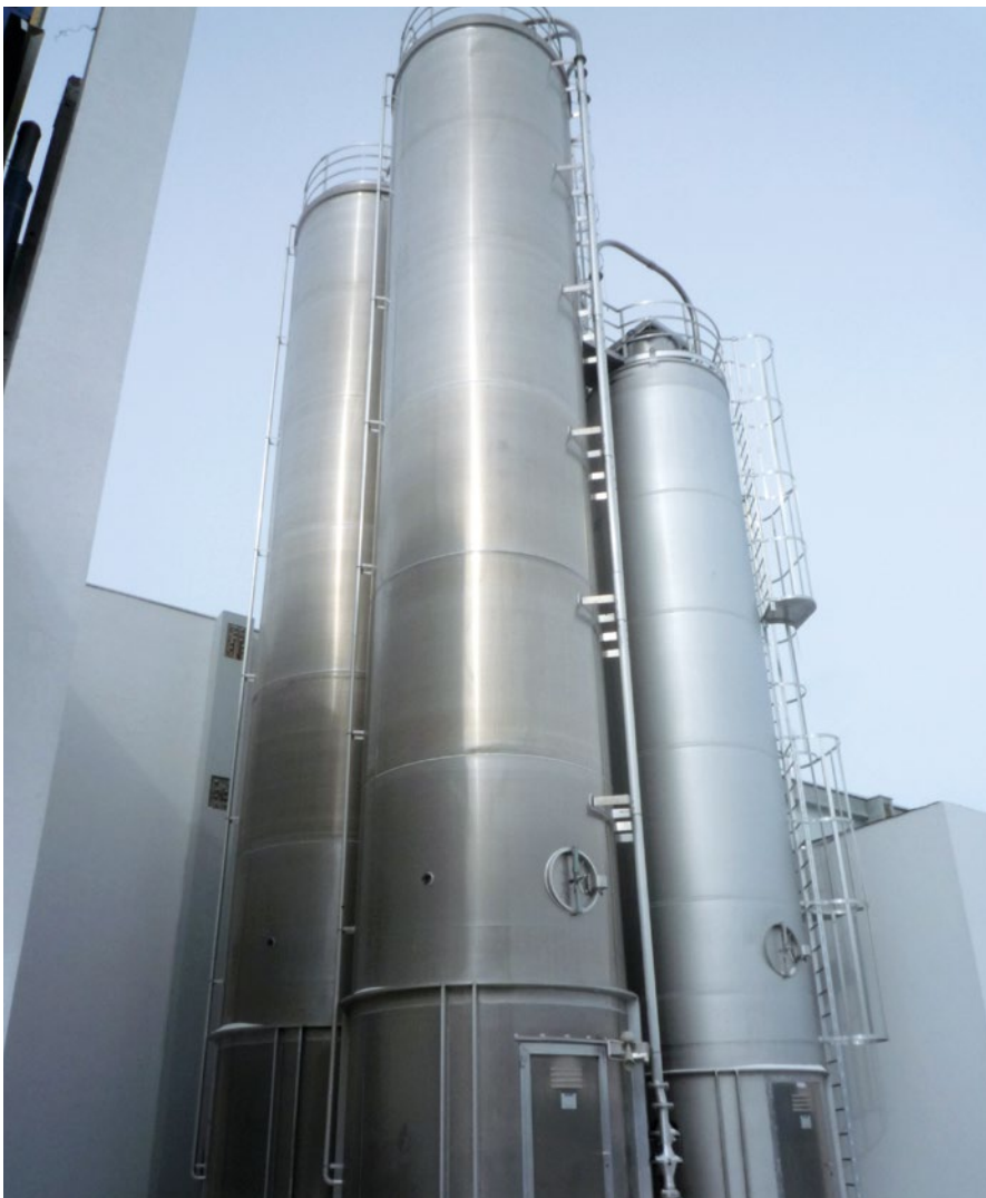
The 30-ton sugar silo and the three 50-ton flour silos are located outside the bakery. The flour for the production is delivered by a mill that belongs to the group.
