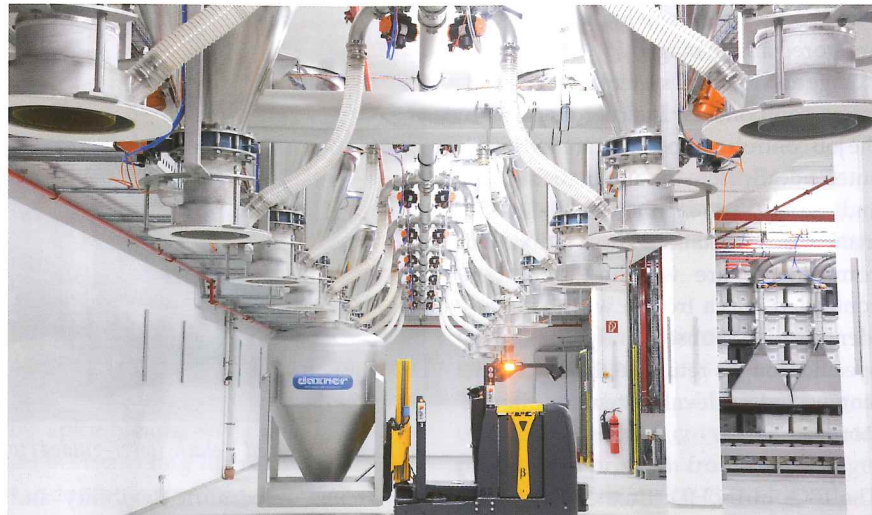
Fully automated collection system with Daxner Container Systems DCS and AGV (Automatic Guided Vehicle)
