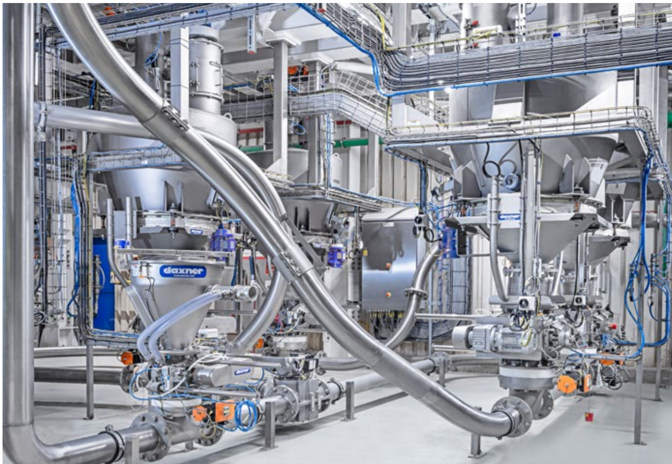
Pneumatic Conveying Systems Fed by Sending Hoppers
