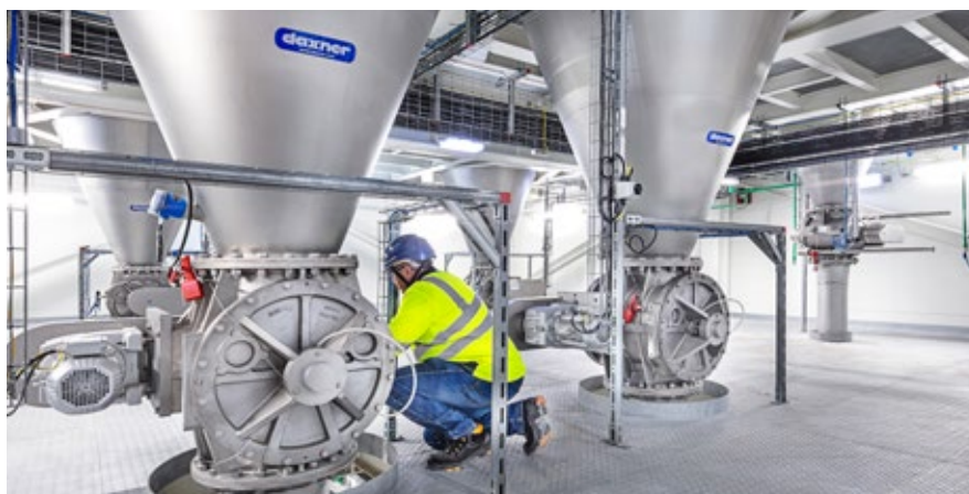
Cyclonic Separators with Rotary Valves
