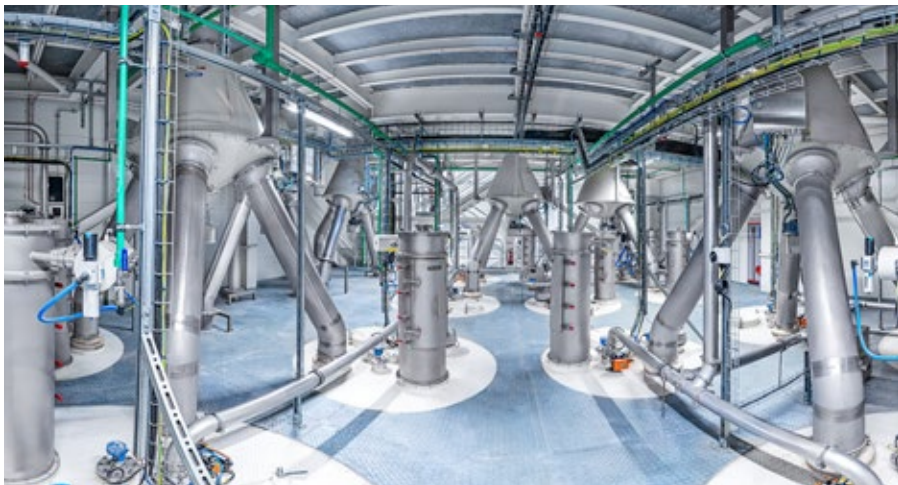
Feeding Raw Materials into the Major Silos
